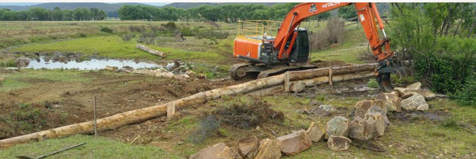
Top: Leaky weir construction at 'Westview' farm, Mulloon Creek, November 2018. Bottom: Same structure after rain, December 2018.
