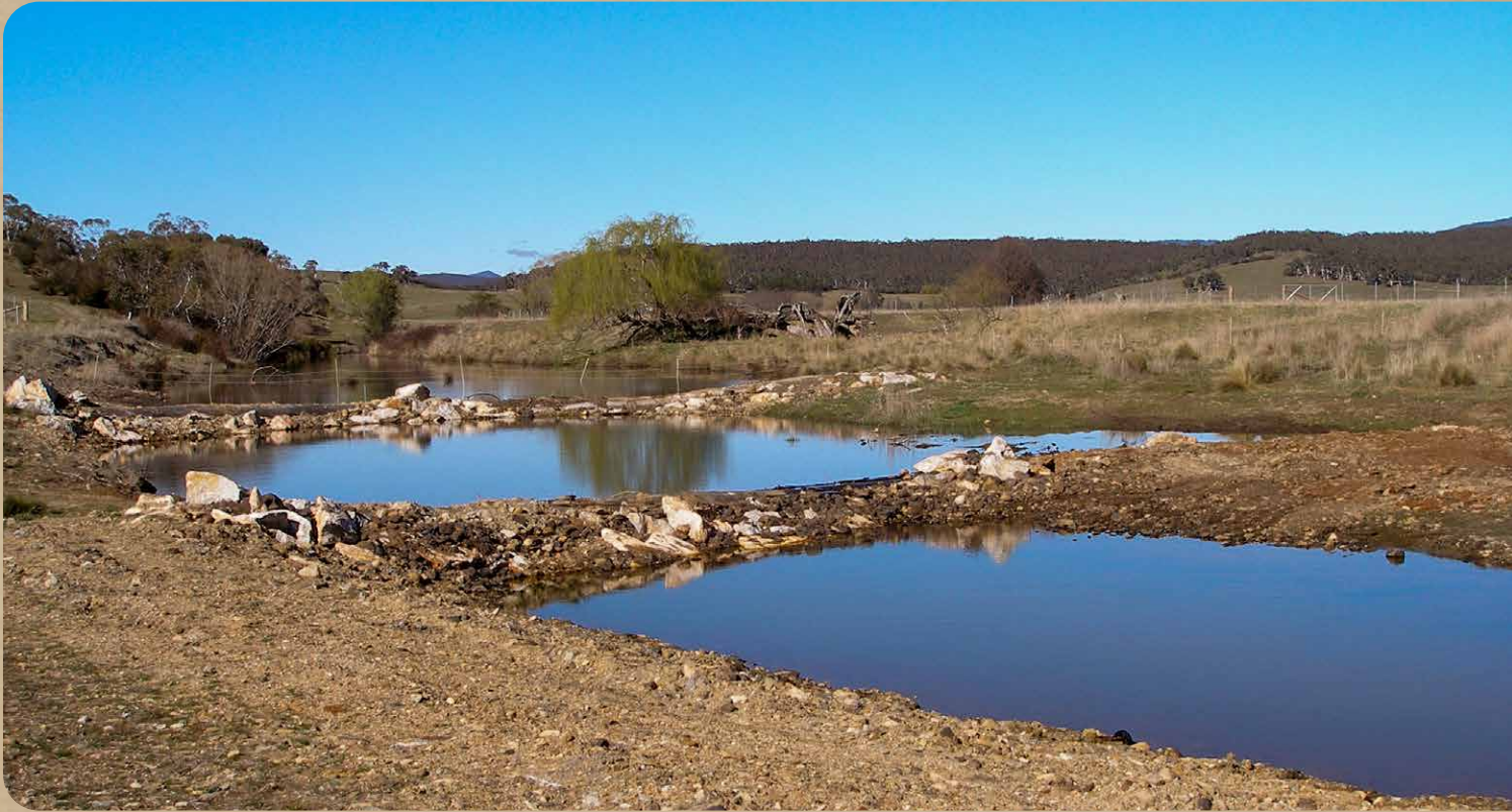
Figure 23: Triple Ponds structure, Mulloon Creek NSW – just after installation in 2006.
