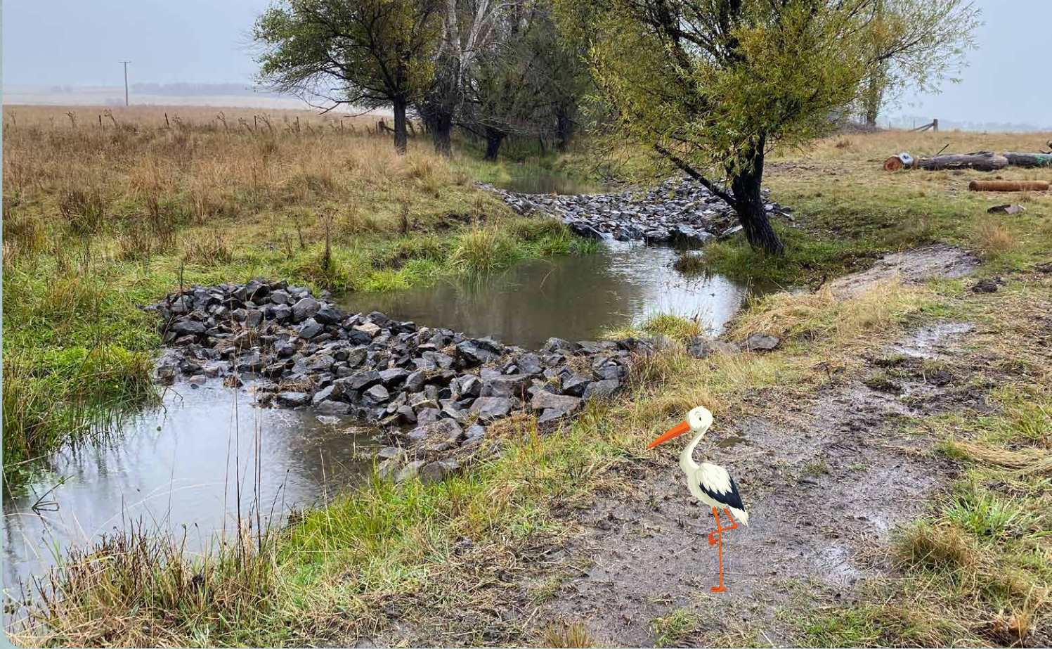
Figure 2: Landscape rehydration infrastructure (leaky weir) installed at 'Lorrina', Braidwood NSW, two days after construction, 2023.
