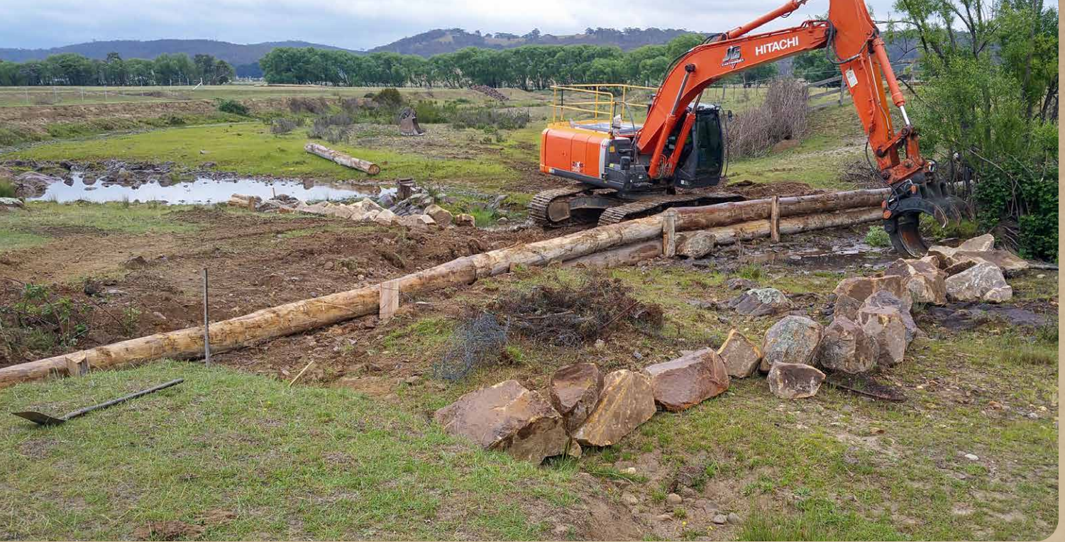
Figure 19: Example of a leaky weir using a log sill structure, under construction at 'Westview', Mulloon NSW, November 2018.
