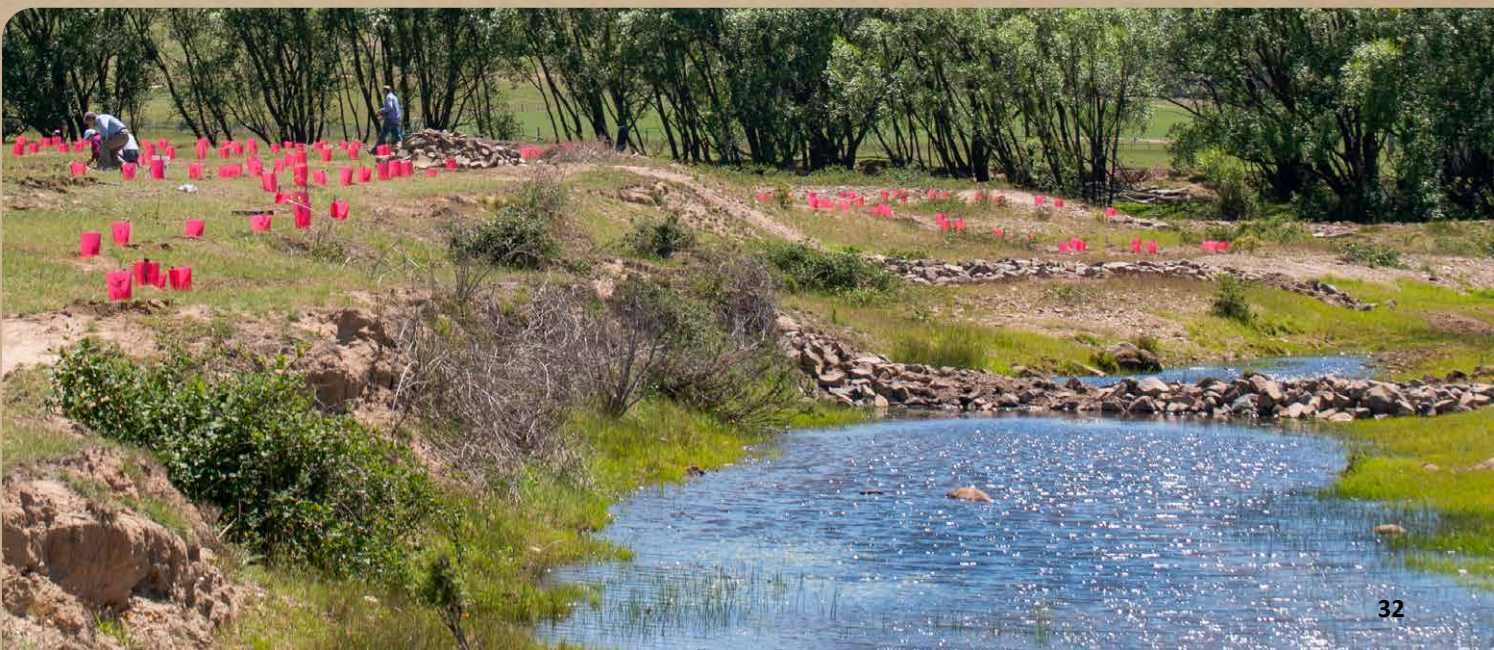
Figure 18: Riparian vegetation being planted alongside leaky weir structures at 'Westview', Mulloon NSW, 2018.
