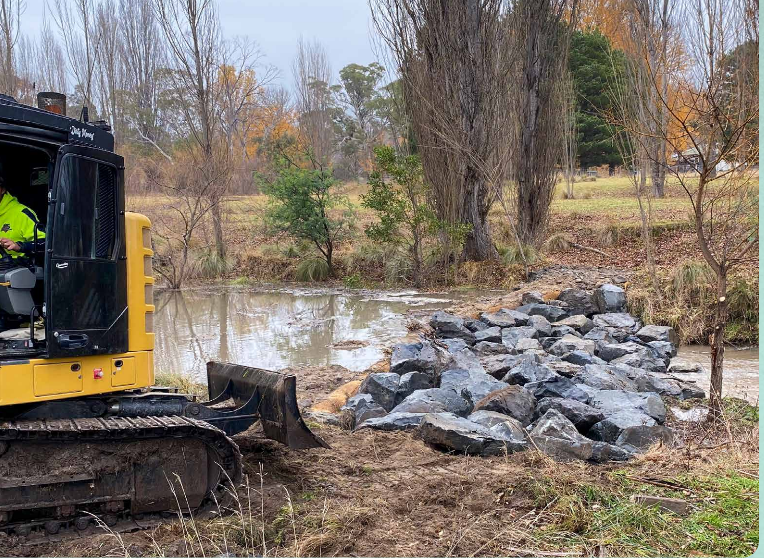
Figure 30: Rocks placed over geofabric in leaky weir at 'Tidbinbilla Station' ACT, 2023.
