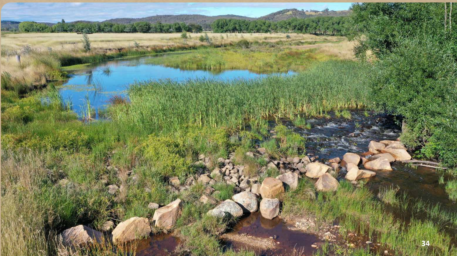
Figure 22: Plants take hold in the rock ramp to provide stability to the structure at 'Westview', Mulloon NSW, December 2020.
