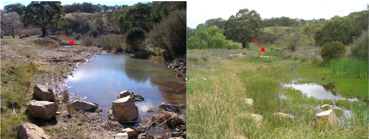
Figure 1.8. View downstream from Weather Station Crossing (LW3) soon after construction, 2006 (left) and Nov 2007 (right). The rock sill is identified by the red arrow. Note the establishment of in-stream vegetation.
